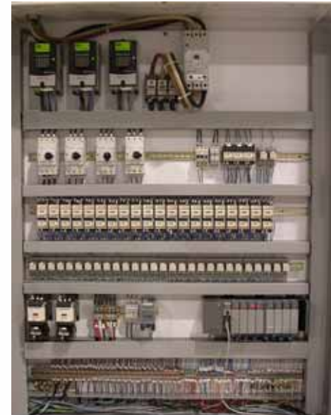
▲ Electrical control panel containing all UL Approved components
